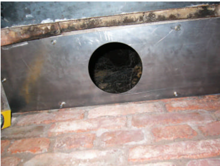
Figure 4. The register plate fitted into the hearth.
